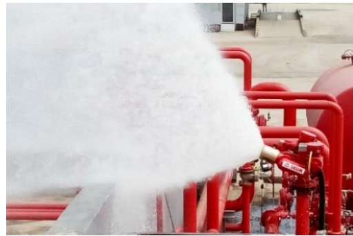
Foam System Package Smart Refinery-Tarjun
