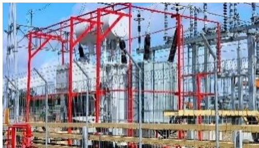
Fire Protection Package PT. PP (Persero) Tbk - Portsite Dual Fuel Power Plant PT Freeport
