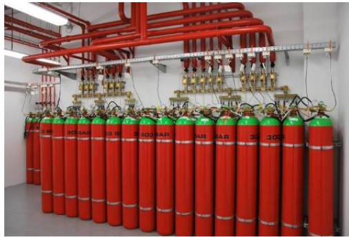
Inergen Fire Suppression System Bank Indonesia, Data Center Kebon Sirih
