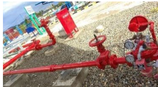
Fire Fighting System Package PT. PP (Persero)-PLTMG Sorong
