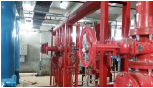
Fire Suppression & Fire Fighting Package PT Berca Hardayaperkasa Phase 1 Site Data Center Indokeppel
