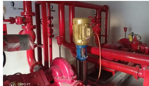
Hydrant & Fire Alarm System Mortar Utama – Semarang Plant
