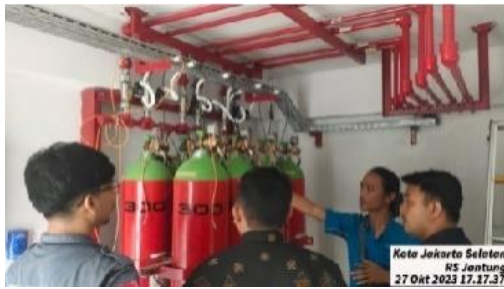
Inergen Fire Suppression Inergen System PT Jaya Kencana RS Jantung Kebayoran Baru
