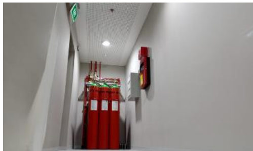
Inergen Fire Suppression System PT Bank Central Asia Tbk. Wisma Slipi
