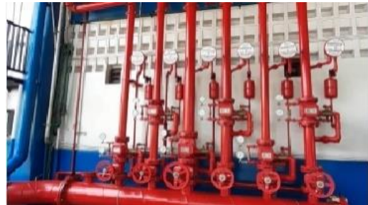
Fire Hydrant System PT. Frisian Flag Indonesia-Pasar Rebo
